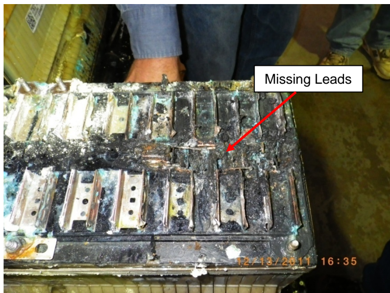
Figure 7.17 – Fire Damage to the Bus Bar Leads
