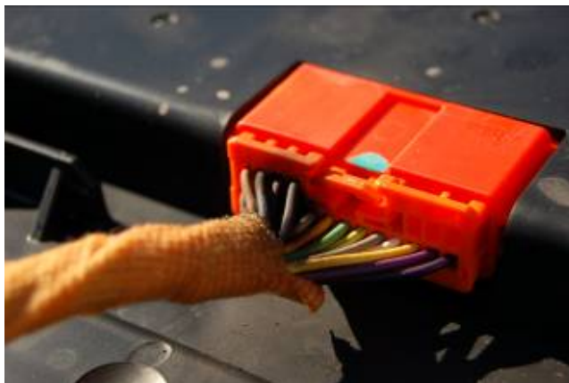
Figure 7.12 – Discoloration of wires and orange jacket
