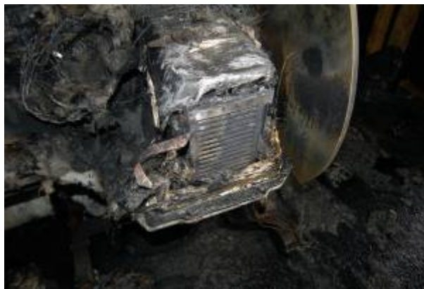
Figure 7.7 – Photograph Showing Cover Damage on the Driver's Side end of Module 3
