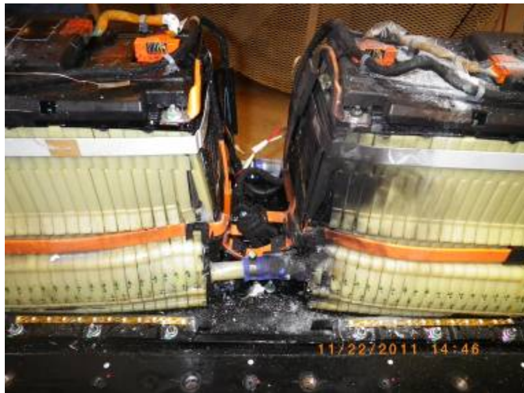
Figure 7.15 – Arcing Damage to the Front of Module 2
