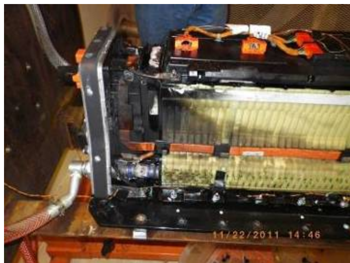
Figure 7.13 – Arcing Damage to the Front of Module 1
